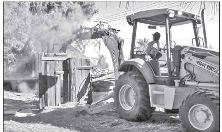
Michael Duwyenie uses a backhoe to tear down the walls of what remained of a long vacant house on Sapphire Lane. QUECHAN NEWS Photo by William Isbell
