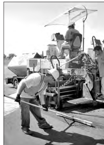
The new gutters between ADAPP and the Wellness Center involved a lot of detail work to get right.
