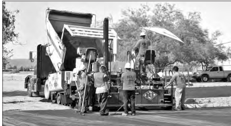
A crew from Desert Road Builders spent the better part of Friday afternoon on August 24th using an automatic paving machine to lay down a thick, asphalt based parking lot inside newly installed curbs. QUECHAN NEWS Photos by William Isbell
