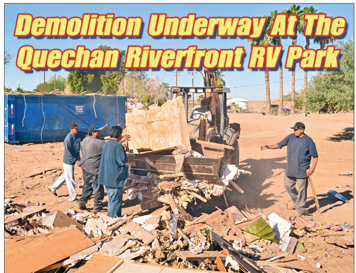
Demolition Underway At The Quechan Riverfront RV Park New environmental regulations mean that rebuilding the water supply and septic systems for the Tribe’s Riverfront RV Park (just south of the Laguna Dam) will have to be undertaken soon, to protect the Colorado River from drainage at the park’s east edge. Rather than attempting a “piecemeal” reconstruction of this important part of the reservation’s infrastructure, the Tribal Council has approved the complete demolition of the RV park, to rebuild the area’s water system literally from the ground up. Taking out the old buildings are Tribal members Luther Emerson, Joshua Golding, Terry Rose, Claude Thundercloud (driving the backhoe) and Felix Montague. The entire project may take up to 24 months. QUECHAN NEWS Photo by William Isbell
