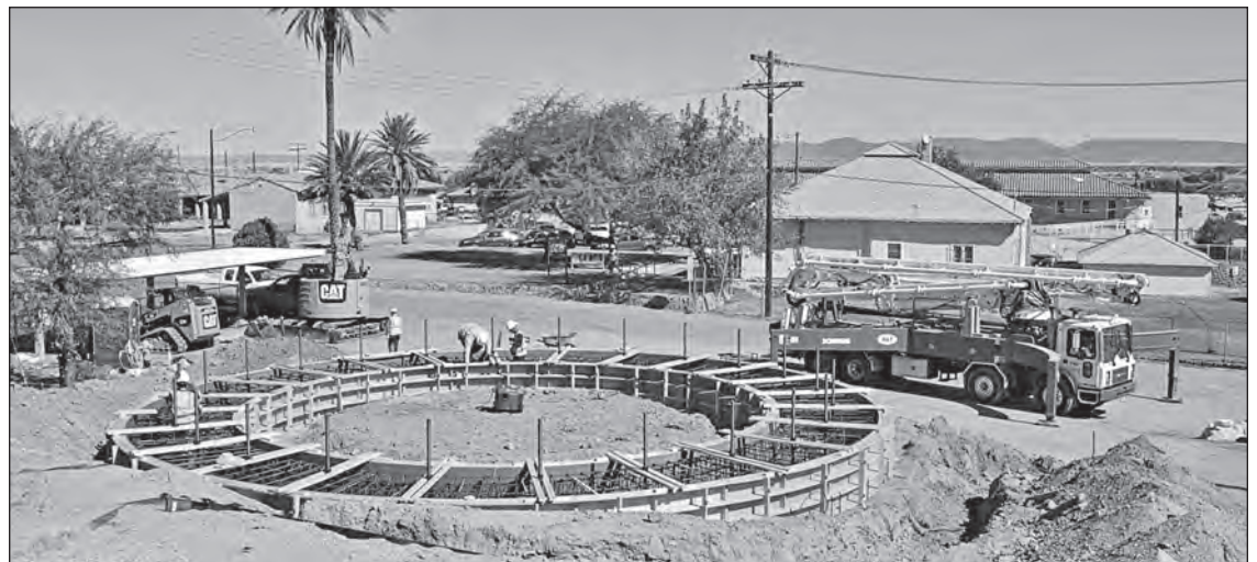
The first group of construction contractors arrived on September 23rd, to at last begin the actual work of building a new, additional water tank on Indian Hill. The first step, levelling the site and laying out markings to indicate where the 40-foot diameter foundation will be placed, was completed within a week. Soil compaction tests were then performed, and an intricate web of steel reinforcing bars tied together in preparation for pouring high strength concrete the following week. Construction of the tank, in the area between the QPD Building and IHS Administration Office, is expected to be completed in February of 2014. Photo by William Isbell
