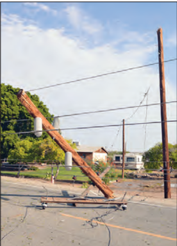
This pole just north of Jimbo's Towing in Winterhaven split in two about 24 feet off the ground.
