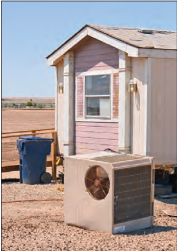
About a quarter mile farther north, Tribal member Milson Jose had the air conditioner torn from his roof.
