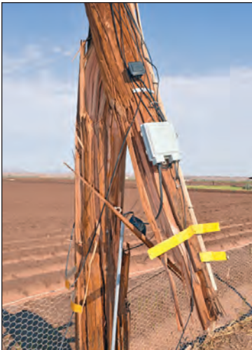
This power pole on Picacho Road managed to stay mostly upright, despite the wind damage.
