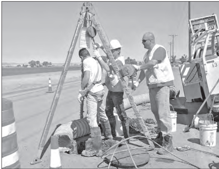
Tyler Morrow (center) and Mike Kiputh of JPCI Services of Mesa, Arizona prepare to lower their co-worker, James Fitzpatrick, into a manhole on Picacho Road. They made up one crew of several performing long needed maintenance on the water drains here on the reservation.
