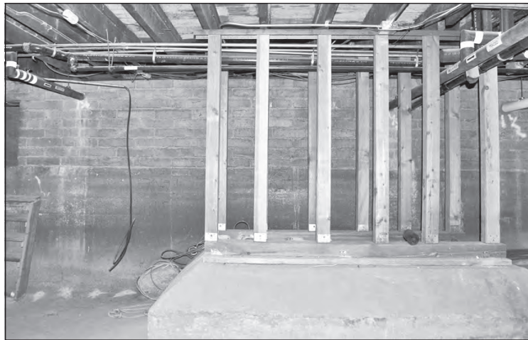
This wooden brace holding up a portion of a wing of the Fort Yuma IHS Clinic is one of the images sent to Congress showing the dangerous conditions that currently exist. QUECHAN NEWS Photo by William Isbell
