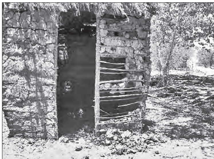
Vandals used a large rock and a tree limb to punch holes through the front wall of the mud hut in early July. EDA Photo by Allyson Collins
