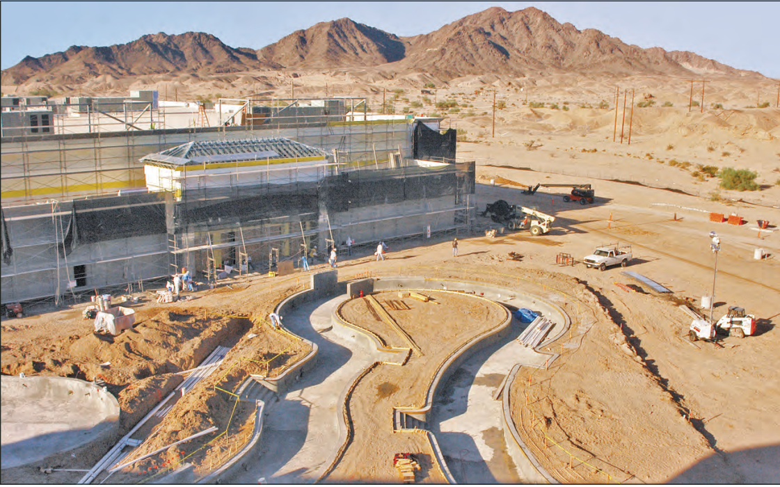
The lazy river water feature is essentially finished and the manifold system that circulates water to the jets can be seen in the trench in the photo above. Angled metal roof beams can also be seen above the entrance to the events center, with the piers for one of the bridges over the lazy river just outside its doors.
