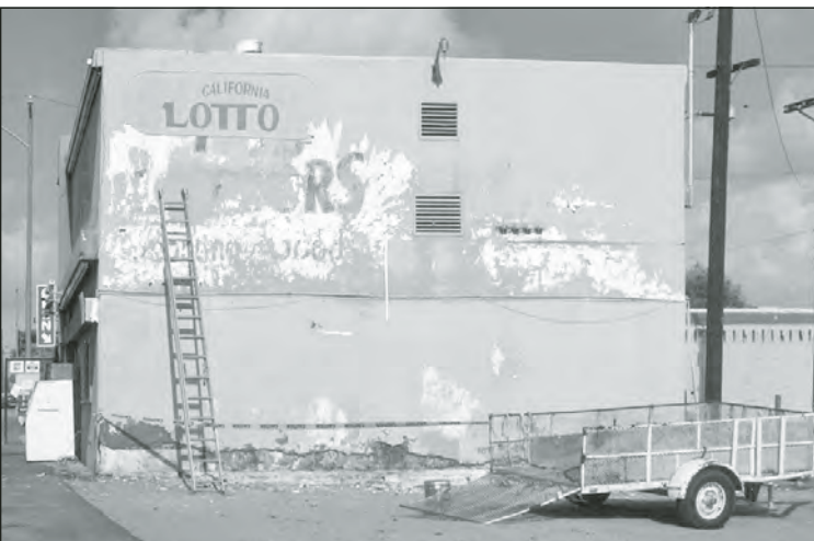
Prior to the facelift , the paint crew from Lima Construction sand blasted the entire exterior of the building to remove loose paint and patched and sealed the cracks and rough spots to give the new paint a smooth surface to adhere to.
