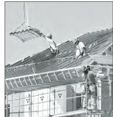
Even during the barbeque, work continued outside, with the installation of the roof frame and steel panels over the elevator tower.
