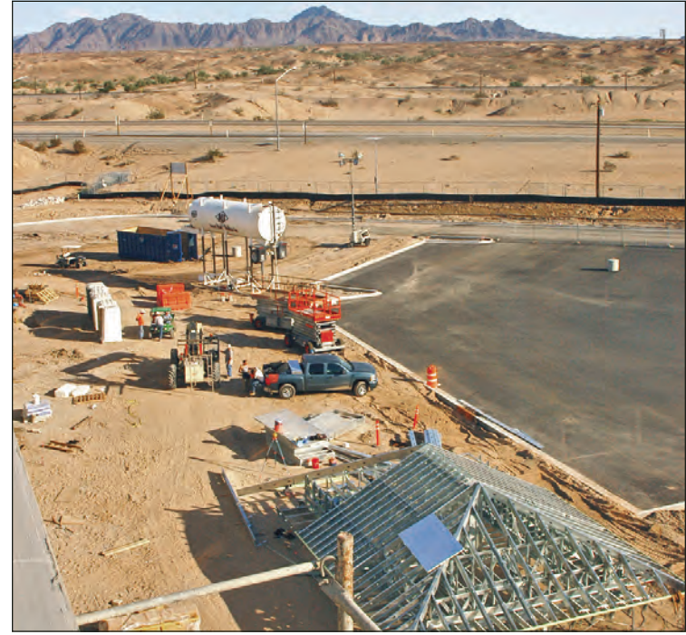
A giant video sign five stories tall will be installed north of the dark blue dumpster, inside the fence at the northwest corner of the property. The roof for the elevator tower is also being assembled nearby.
