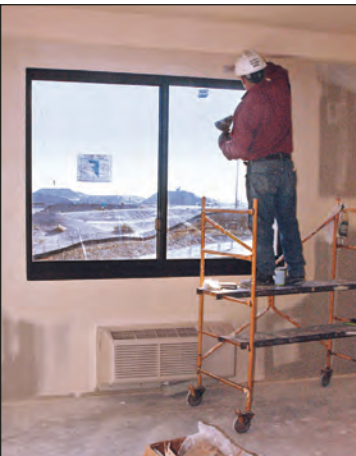
Hotel rooms are being finished and painted from the top floors down. Tile work is already being installed in the guest bathrooms.
