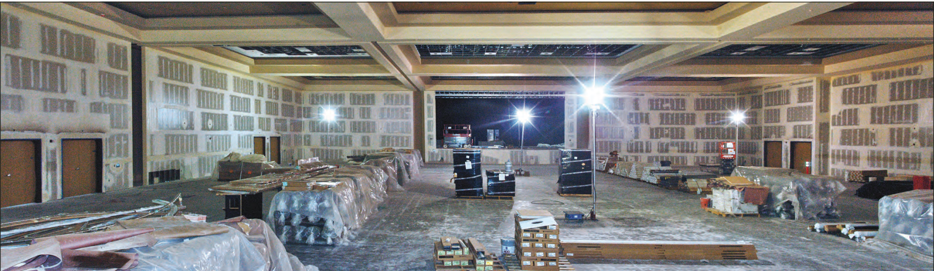
The Events Center Stage is seen surrounded by portable sodium vapor lamps and various supplies being stored for later installation in all areas of the complex. The large light colored box-beams in the ceiling contain the overhead tracks for portable walls on either side of the stage. Two long moveable walls are also installed in pockets on both sides of the double doors to the left. The walls enable the events center to be subdivided into six rooms with a central hall for separate meetings at the same or related events.
