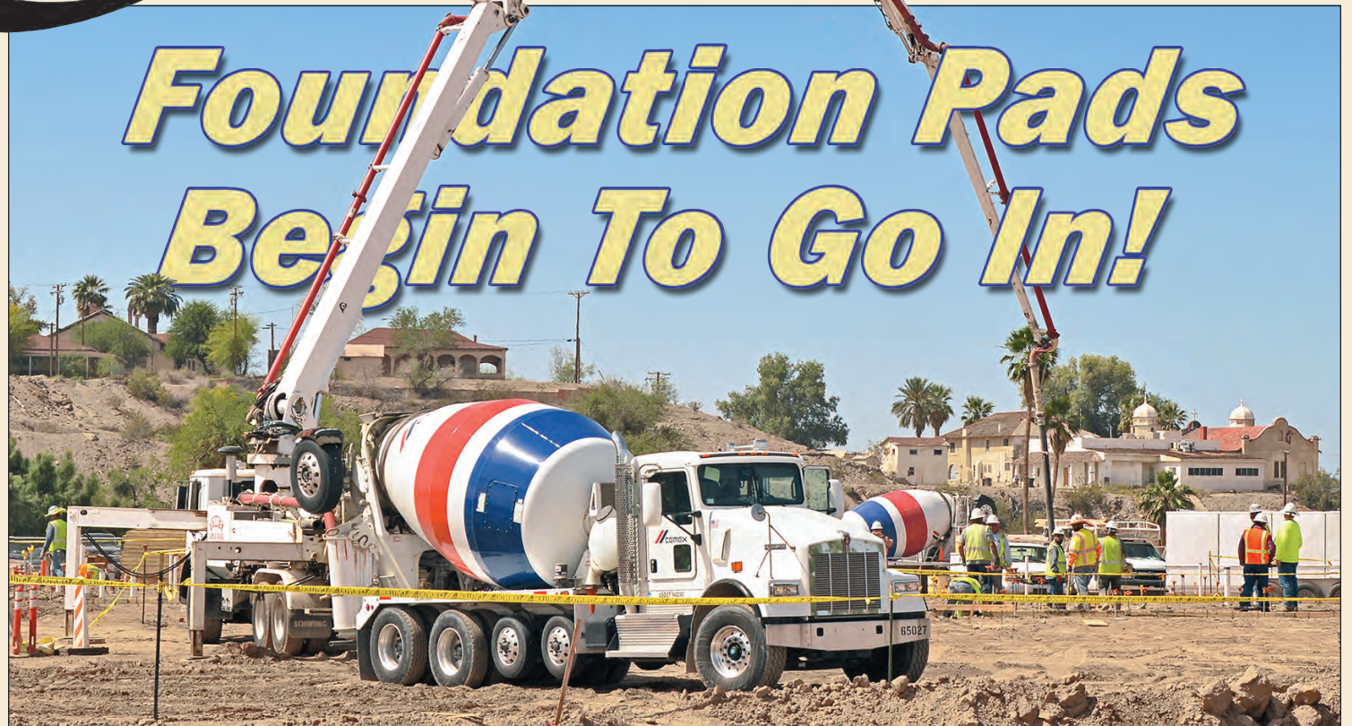
Concrete began to flow into the footings for the new Fort Yuma Health Care Center's Building A on Thursday, May 5th, under the watchful eye of the on-site superintendents working for Pilkington Construction, the general contractor on the 20 month project. Quechan News Photo by William Isbell
