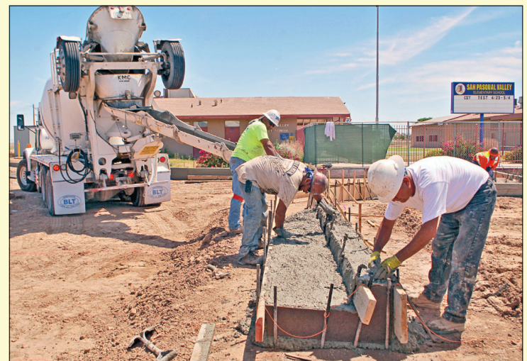
Team C Construction employees Tomas Romero, Jacinto Piña and José Saravia (in the foreground) from El Cajon work on pouring and smoothing new curbs for an all new driveway going in north of the elementary school office.
