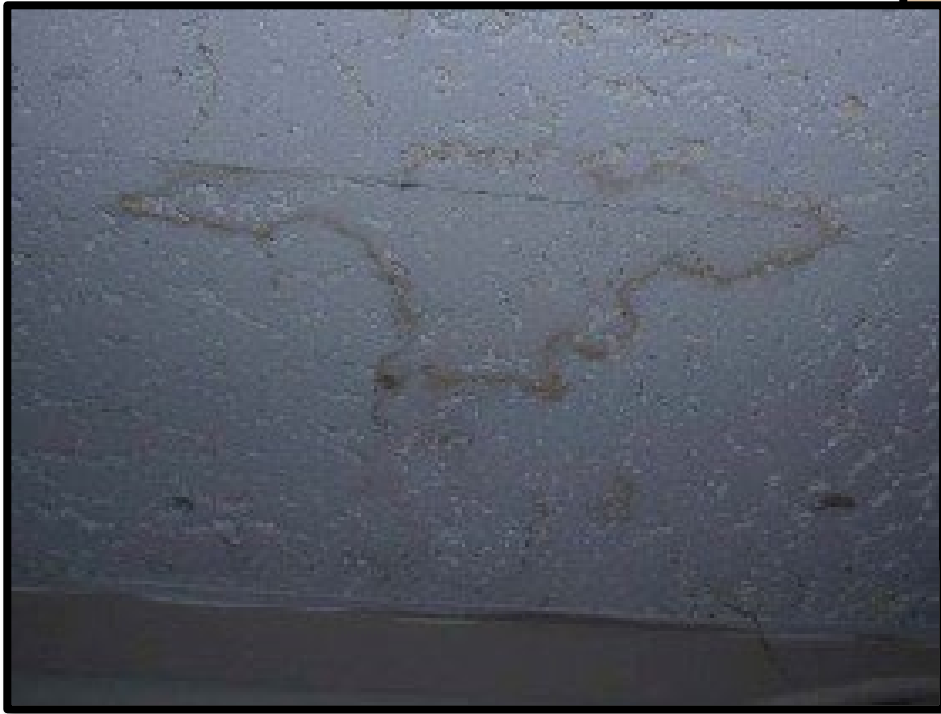
Rodent urine stain in dropped ceiling
